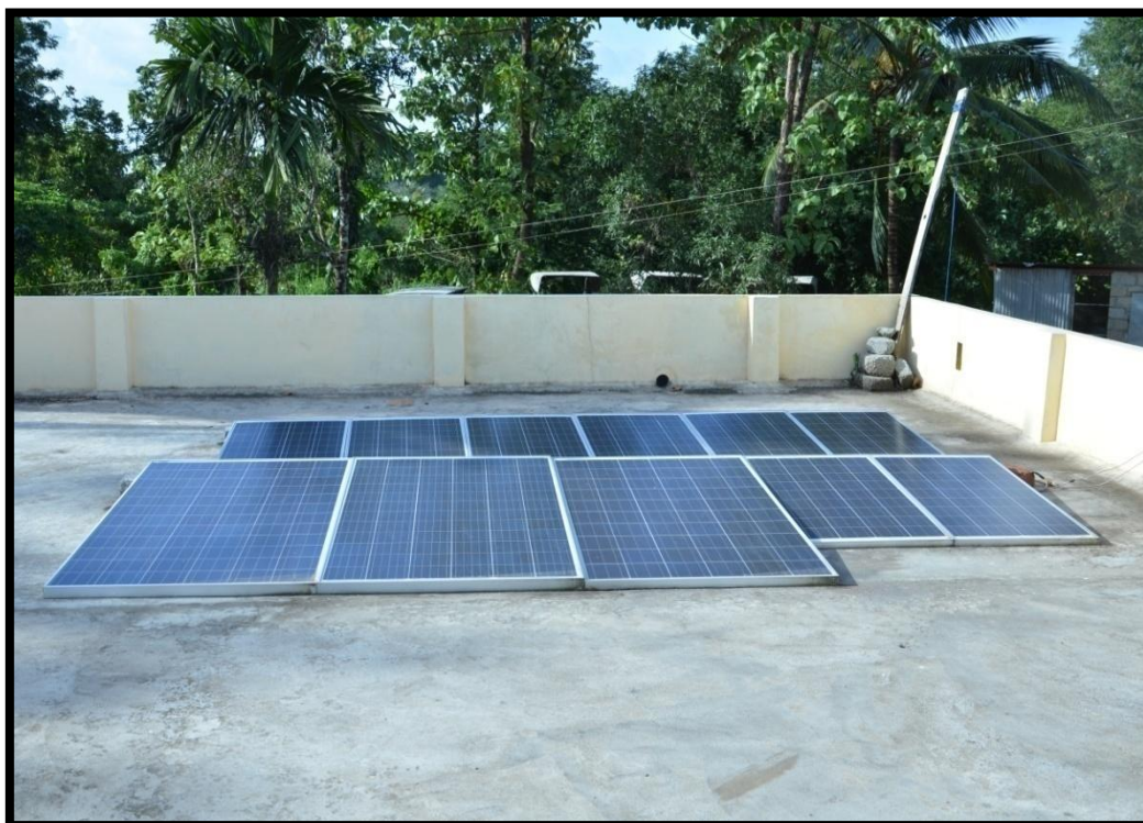
Solar panels for office
