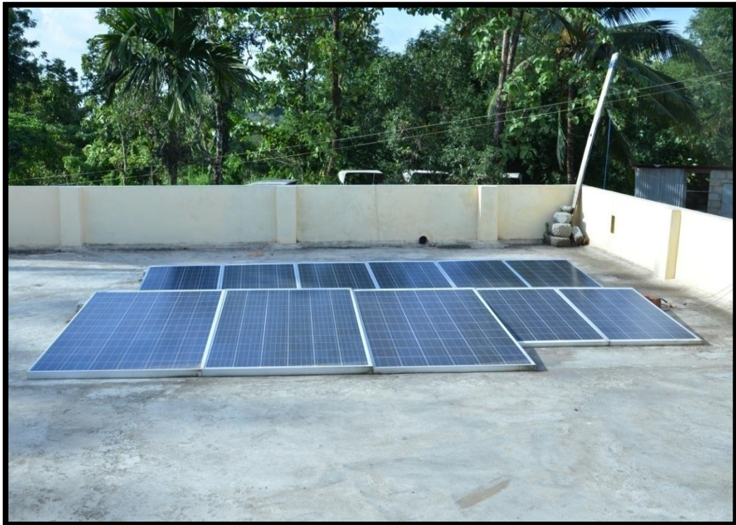
Solar panels for office
