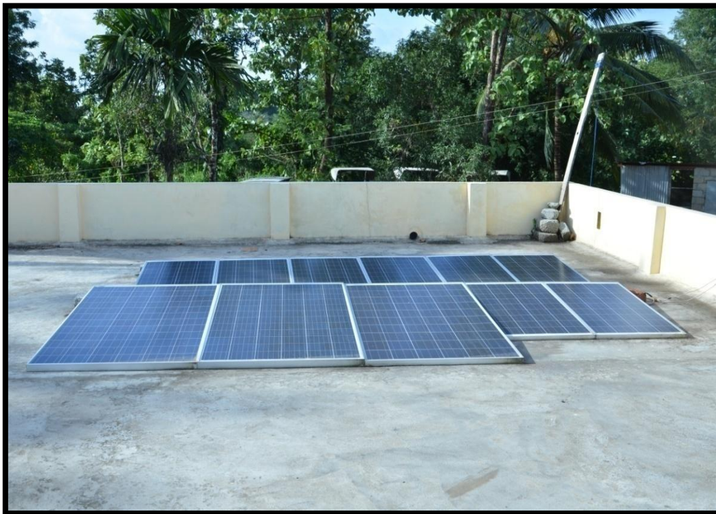
Solar panels for office
