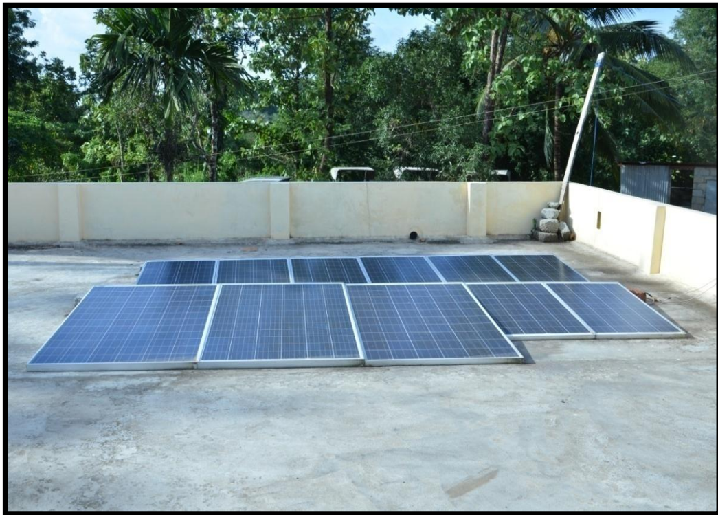
Solar panels for office
