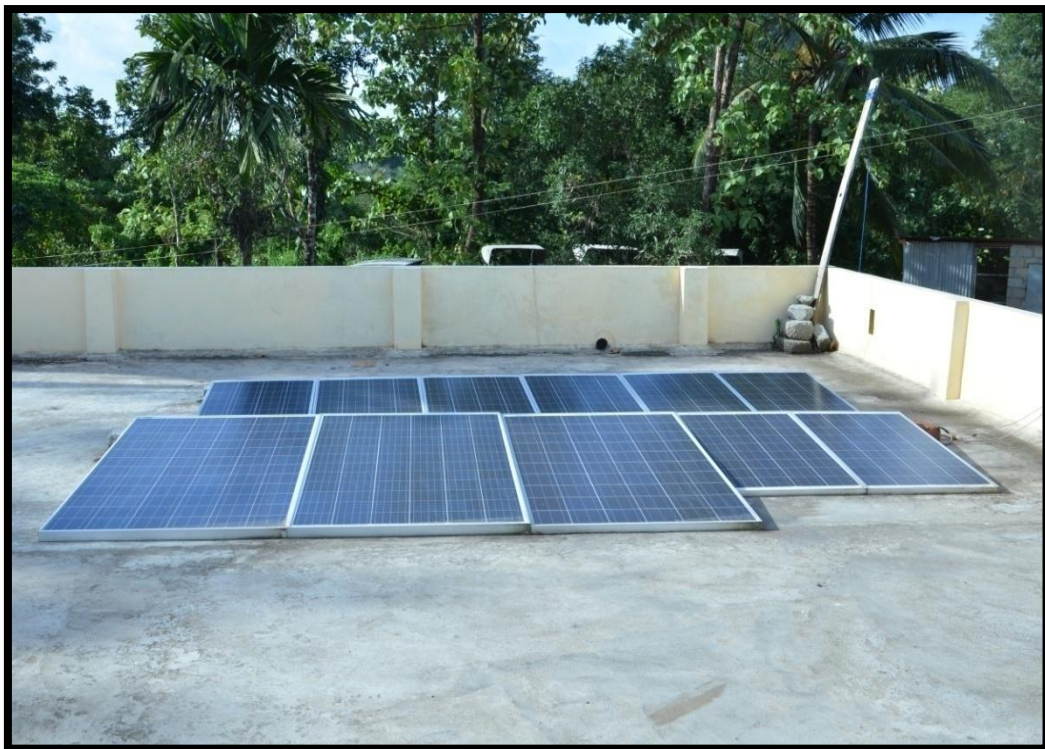
Solar panels for office
