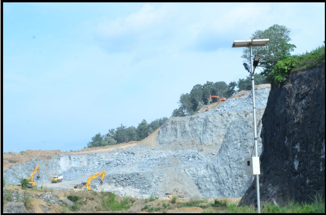
Solar Street light
