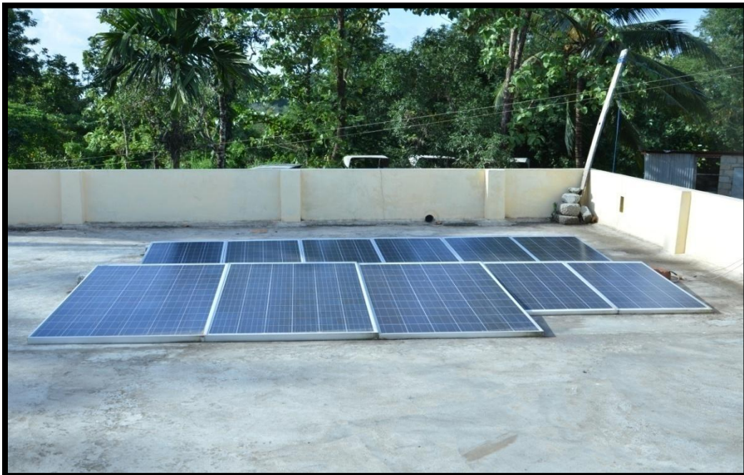
Solar panels for office
