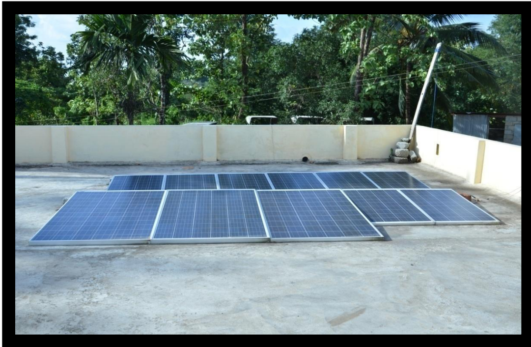
Solar panels for office
