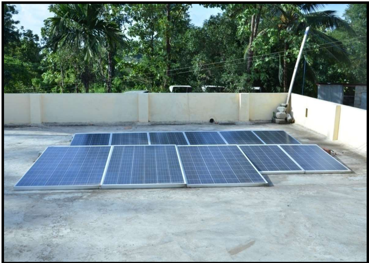
Solar Street light/panels
