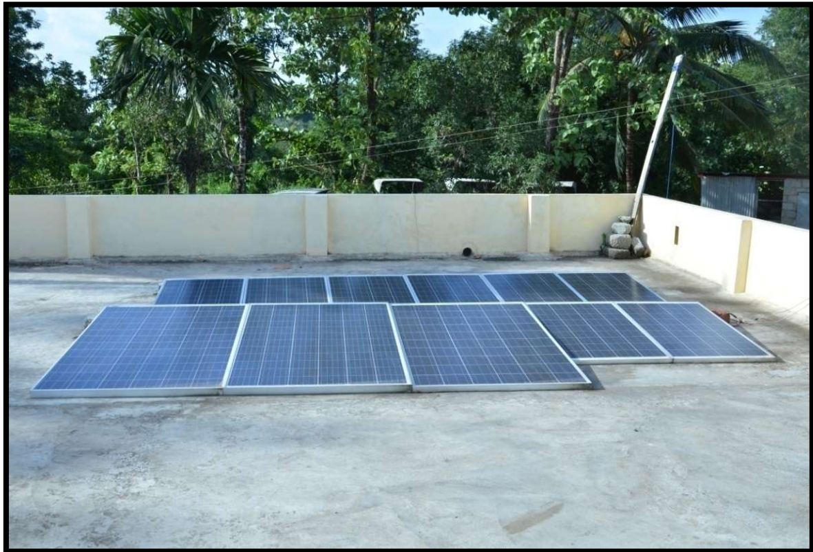
Solar Street light/panels
