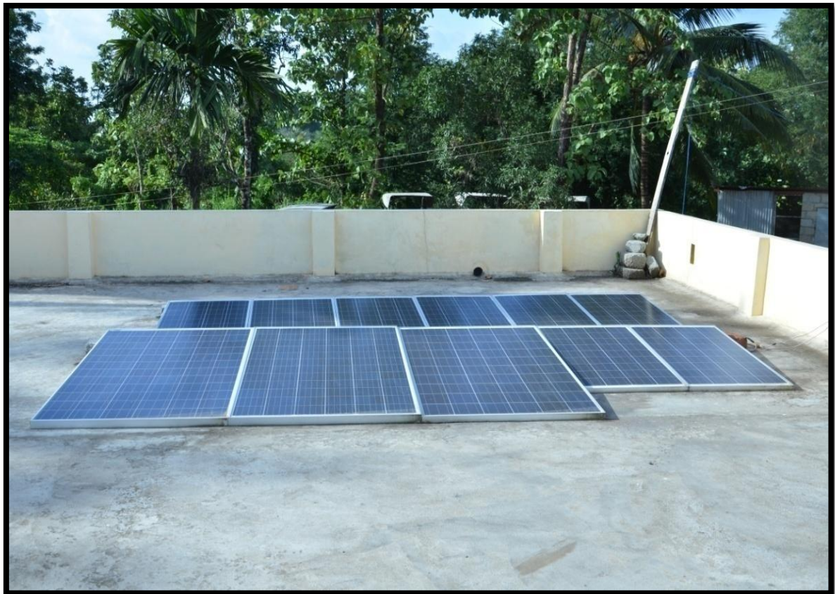
Solar Street light/panels
