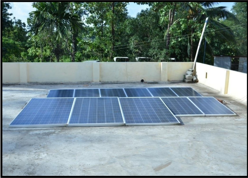
Solar panels for office
