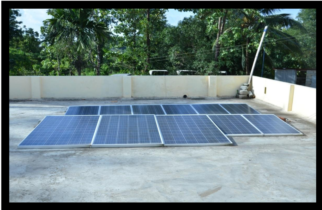
Solar panels for office
